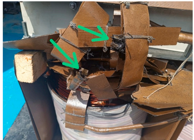
Fig. 11. Thermal fault with hot-spot fault inside the zig-zag transformer.
